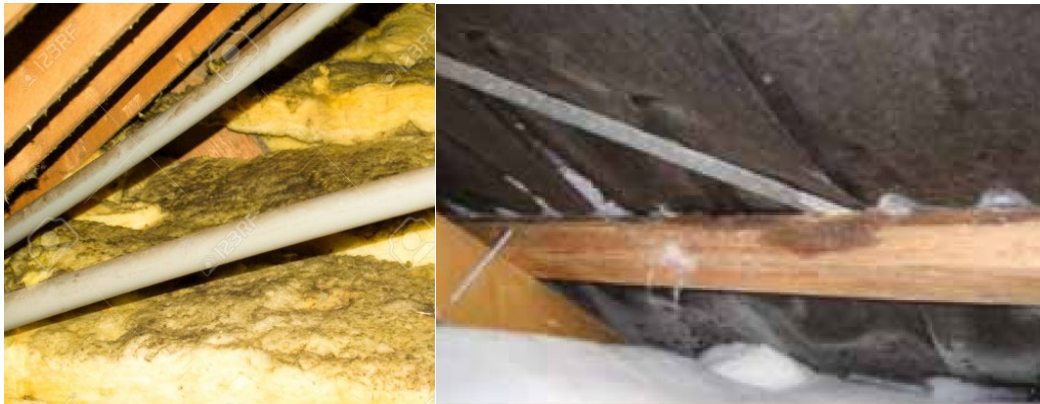
Figure 7. Two common examples of damage caused moisture build-up in an insufficiently vented roof space.
